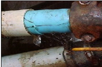
Flexible piping is cracked
