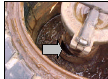
Spill bucket in poor condition – note the gap between the spill bucket and the fill pipe
