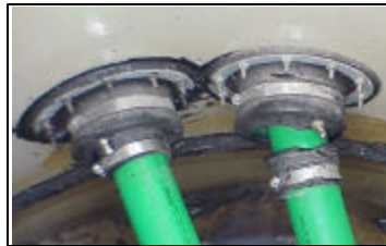
Test boots positioned at sump wall, right test boot is torn
