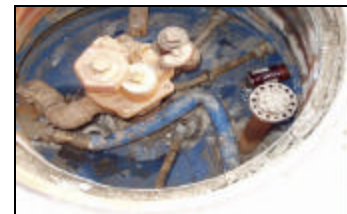
Flexible piping is kinked
