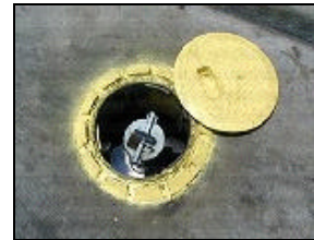
Circular spill bucket lid pulled back to show the fill port with a spill bucket
