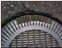
Cracked spill bucket lid
