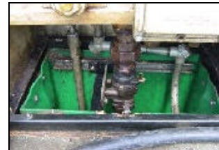
Contained dispenser sump
