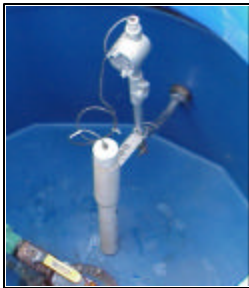
Float sump sensor
