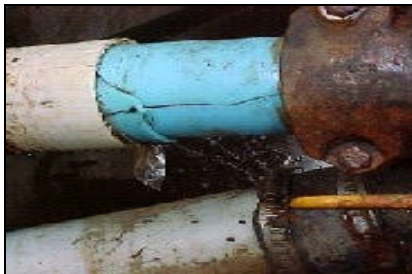
Flexible piping is cracked
