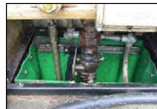
Contained dispenser sump
