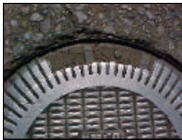
Cracked spill bucket lid
