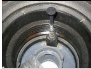
Spill bucket drain valve
