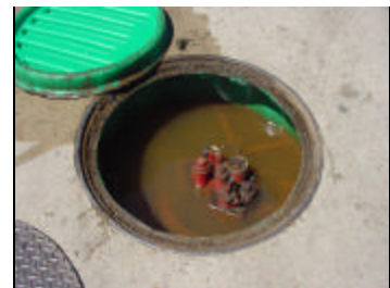
Contained turbine sump full of liquid
