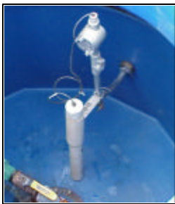
Float sump sensor
