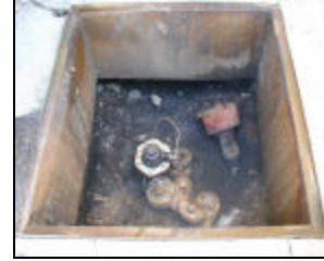
Uncontained turbine sump
