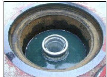
Spill bucket that contains liquid
