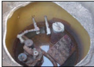
Contained sump with liquid and debris
