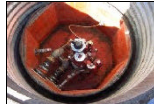
Contained turbine sump
