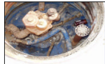
Flexible piping is kinked
