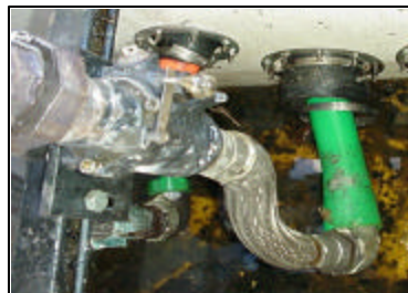
Metal flexible connector is twisted due to growth of flexible plastic piping
