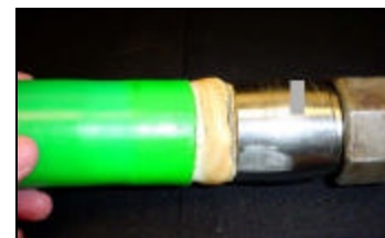
Flexible piping is bulging
