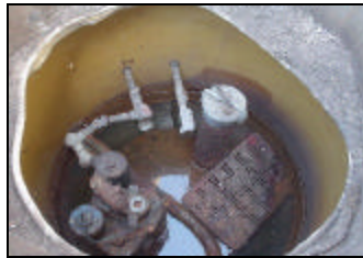
Contained sump with liquid and debris
