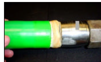
Flexible piping is bulging
