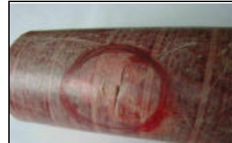
Fiberglass piping is cracked
