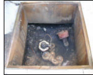
Uncontained turbine sump
