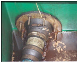
Sump penetration seals in poor condition
