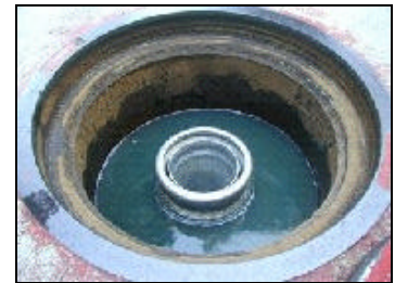
Spill bucket that contains liquid
