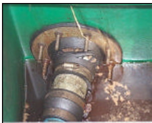
Sump penetration seals in poor condition
